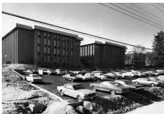
Figure 87 - Construction of the Arthur H. Armstrong (left), Ralph A. Hefner (center) and Hugh H. Caldwell (right) residence halls, October 1969. Georgia Tech Photograph Collection
